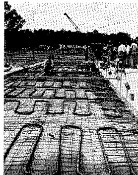
insulating slab of perlite concrete under radiant piping cuts heat loss to ground.
